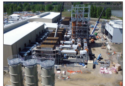
With 12 new natural gas engines (top) at Port Westward in Clatskanie, Oregon (bottom), Unit 2 will be the most efficient simple cycle plant in the U.S.
